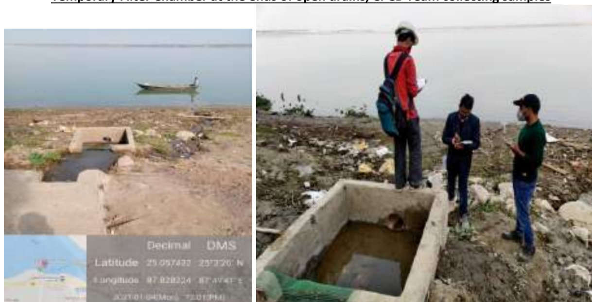
Temporary Filter Chamber at the ends of open drains, CPCB Team collecting samples
